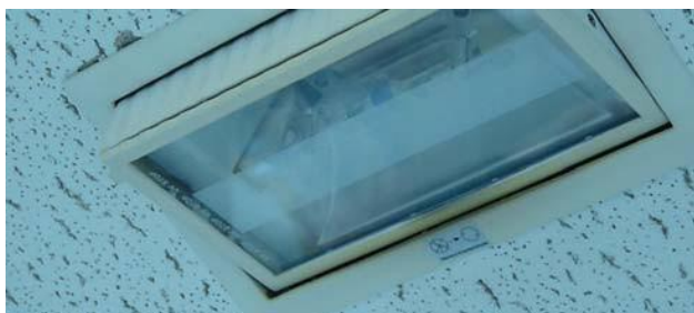
Halogen lighting - signs of overheating & flickering were present
