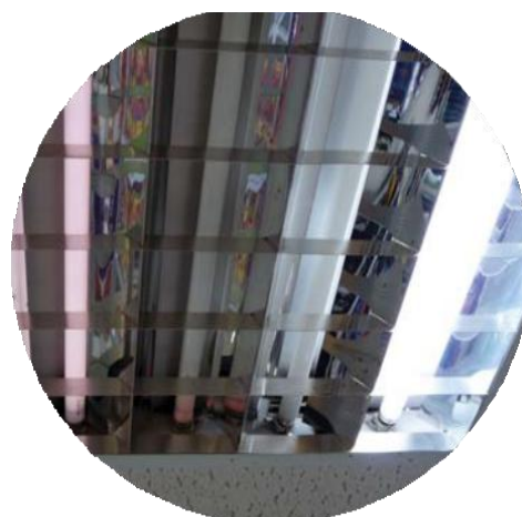
T8 lighting - requiring regular maintenance
