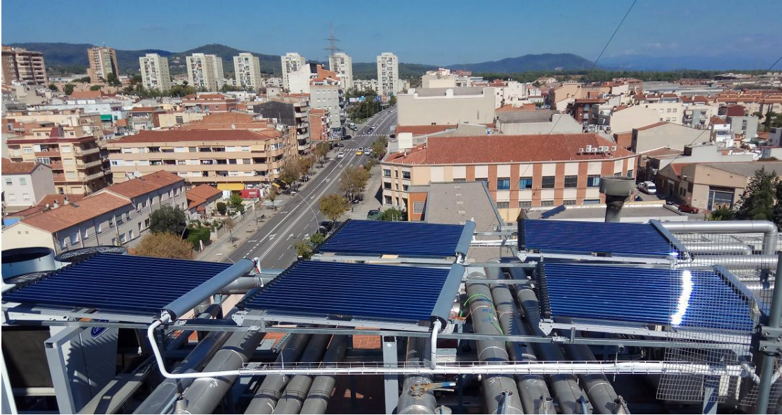
*General view of THERMX solar thermal installation.
