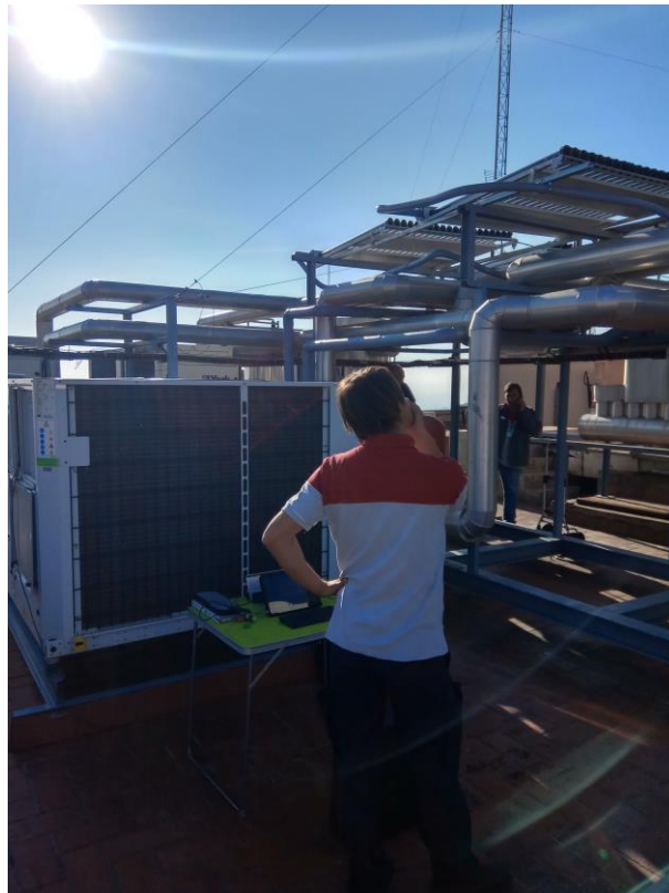
*inspection and control visit of the manufacturer of the HVAC equipment.
