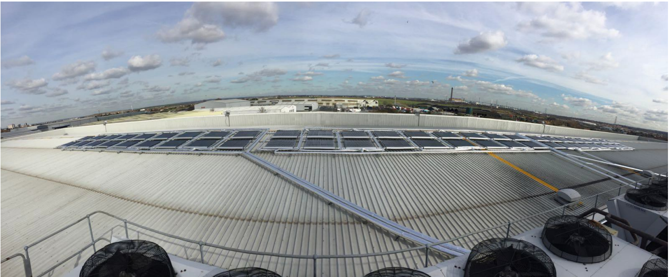
Image 2: the solar thermal collectors installed in parallel on the roof of the Chingford fruit facility. Source SCE picture gallery
